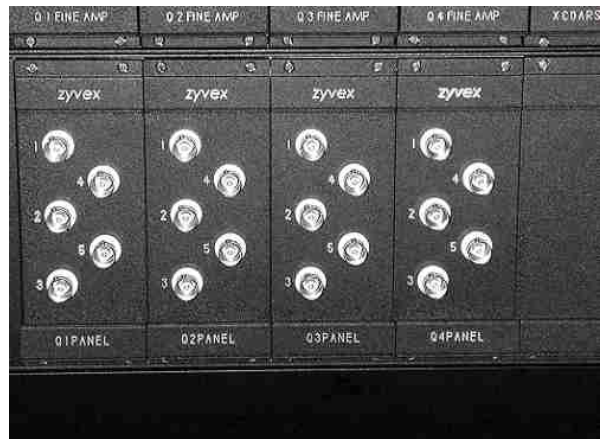
Figure 4 S100 patch panel interface
